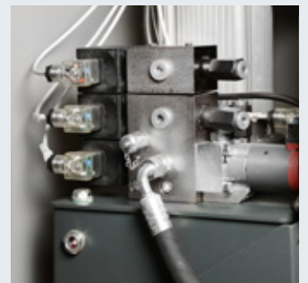
50-C10P/2F upgraded with third electrovalve 50-C10D/3F
